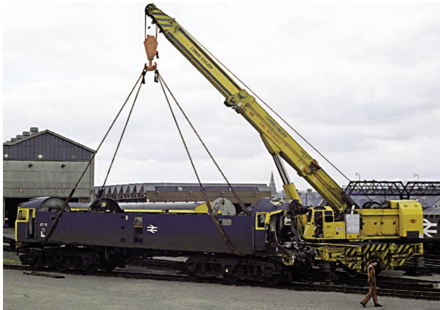
ABOVE: Following the introduction of the Cost Effective Maintenance (CEM) regime, Canton took on the role of carrying out bogie overhaul work for a number of Class 47 locomotives. Traditionally this would have been undertaken at Crewe Works but the CEM regime involved moving a lot of the heavy maintenance work from Main Works to what would become 'Level 5' depots, one of which Canton would become. As part of his role as Technical support Engineer at the depot Brian was responsible for co-ordinating this work. In order to commence the overhauls, the depot needed a 'float' of bogies. These were obtained from crash damaged 47 111 which had been involved in a collision with a DMU in Preston station in January 1986. In this view, with the power unit already removed the loco is in the process of being lifted from its bogies outside Canton depot Main Shed on June 4, 1986. The body would eventually be cut up on site by depot staff before October the following year. Steve Morris
